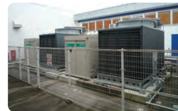
Energy-efficient heat exchanger
